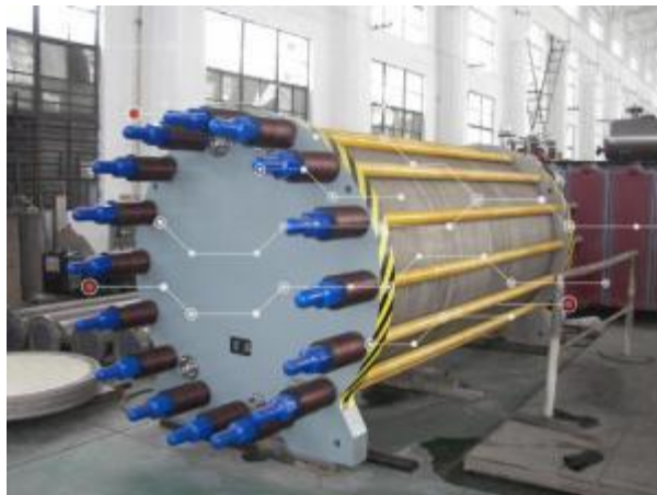
国产1000Nm 3 /h中压水电解制氢装置 A domestic 1000Nm 3 /h medium pressure water electrolysis hydrogen production facility
