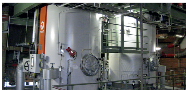
Electrode boilers in the combined heat and power plant at the industrial park, Höchst, Frankfurt Photo: Infraser GmbH & Co. Höchst KG
